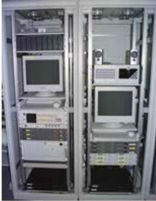
Shared Storage and Server
